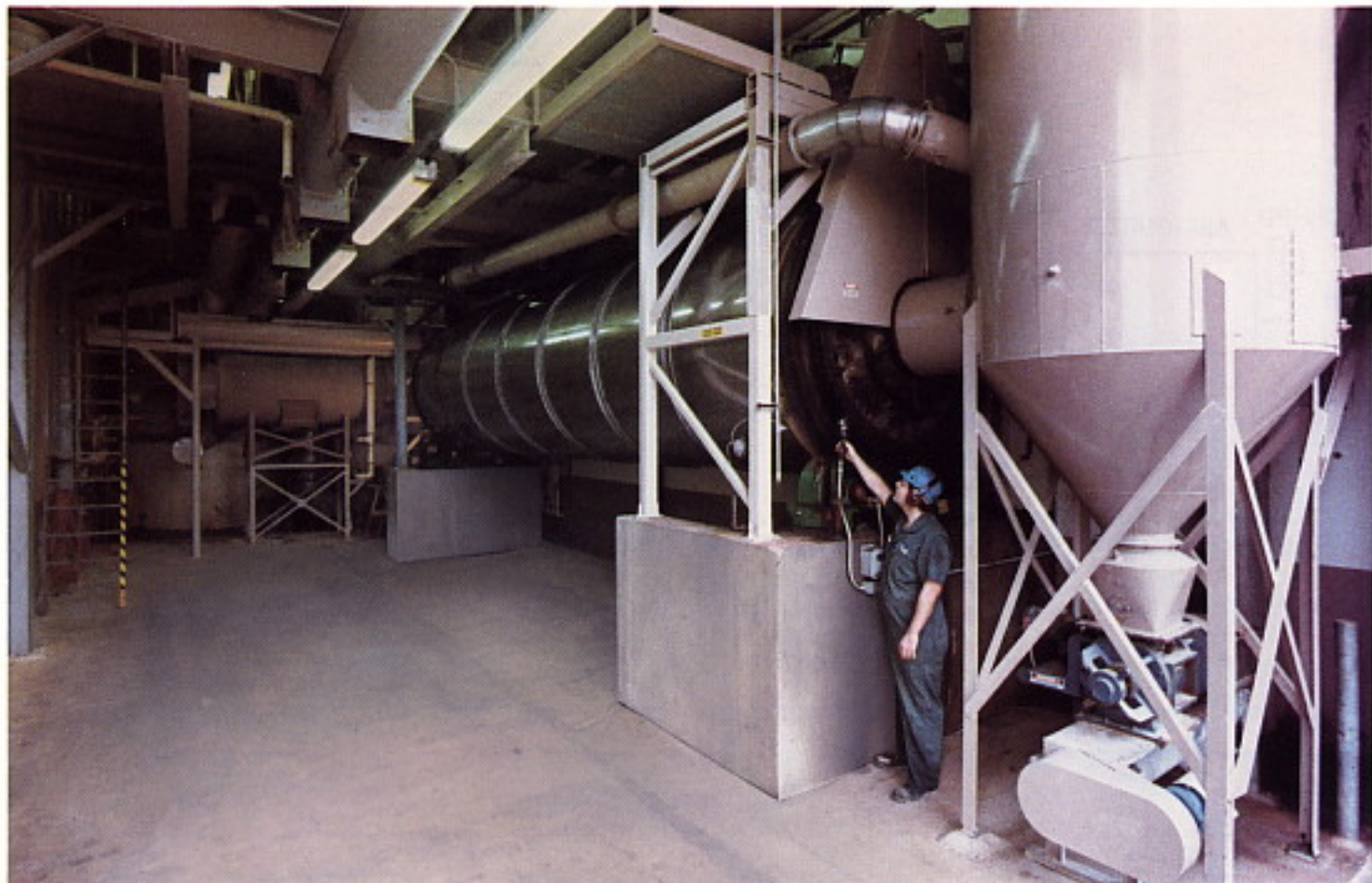
Duske Sludge Dryer System
